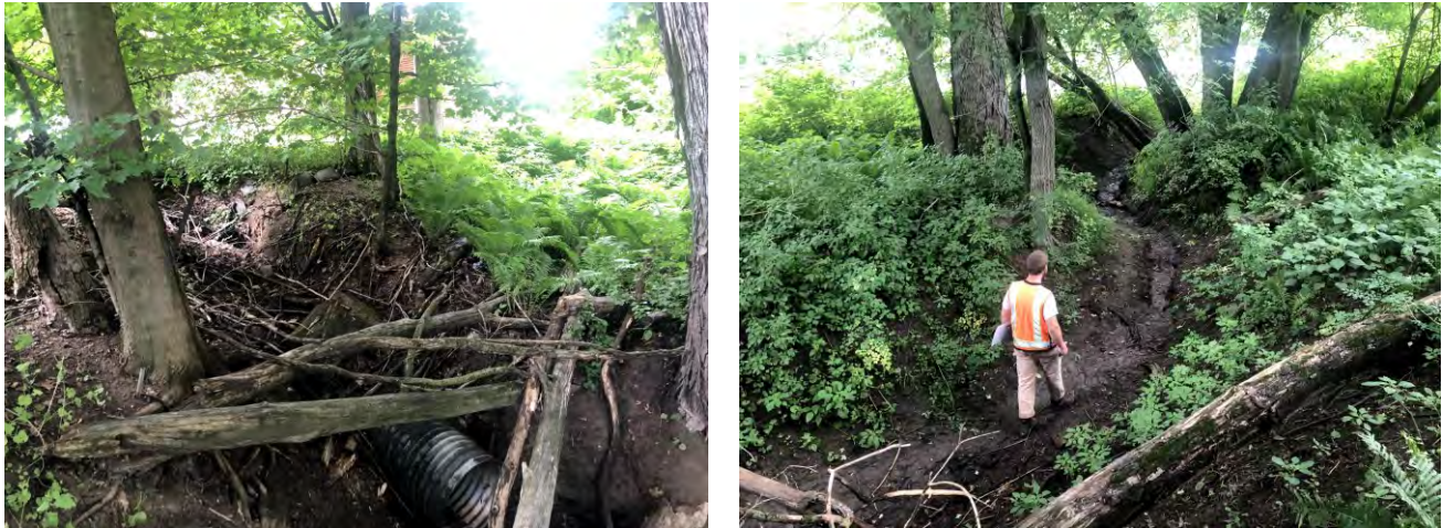
Figure 7: Project CV-11 had the highest score (21 out of 30) in the Non-Unified Prioritization. The project is located at the outlet of a culvert that drains much of the Cambridge Village center. The last segment of the culvert has failed, and a large gully has formed with erosion that extends to the edge of the Lamoille River. When the Lamoille River experiences elevated flow, this gully has been observed to backfill with water. The opportunity to treat a large volume of water and a very high sediment/nutrient load warranted a 10% design for this project.
